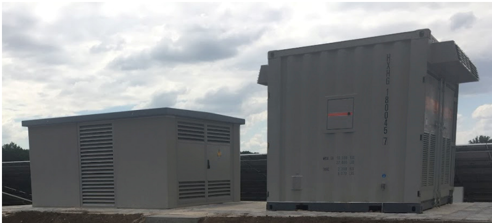
Figuur 10: Impressie transformator/inverterstation
